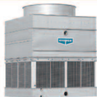
냉각탑 (COOLING TOWER)
